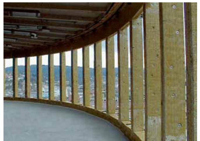
Fire protection sheathing on steel supports
