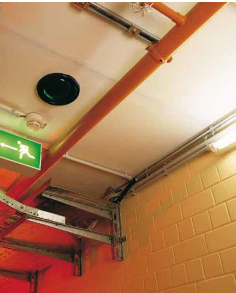
F90 fire-proof ceiling in a service room
