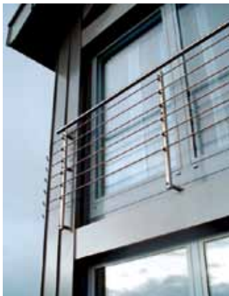
Room-high aluminium window system with outside falling protection on a residential building
